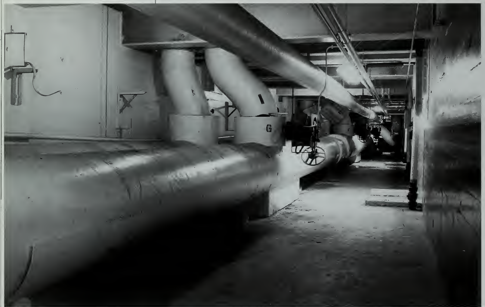
Interior, heating and cooling plant, December 1942
